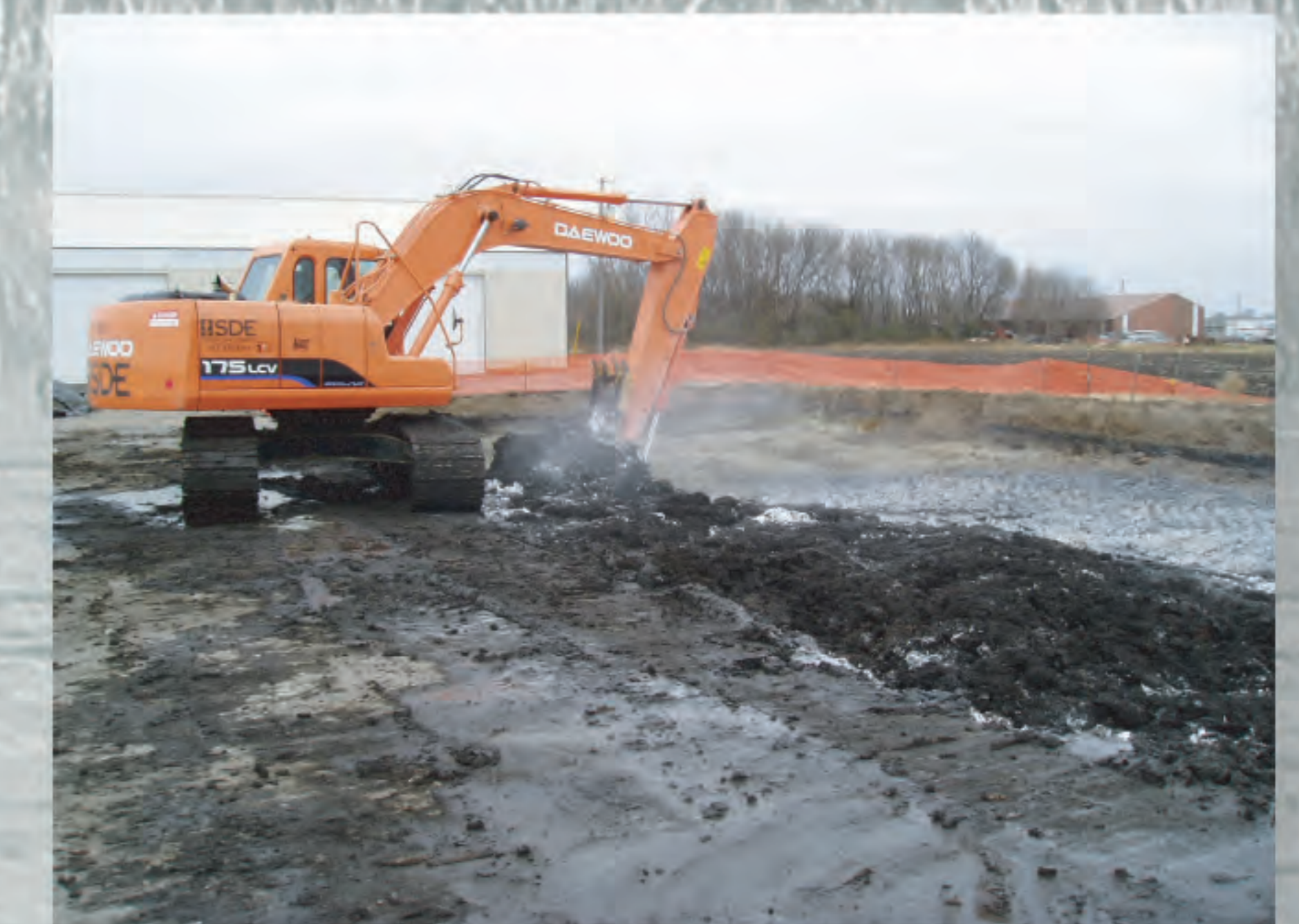
During treatment, 7,000 lb of lime were added to temporarily raise the pH and to reduce the moisture content before landfilling.
