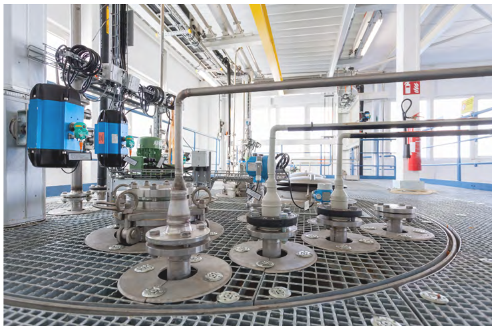
A wastewater treatment plant that uses Eisenmann's proprietary, two-reactor Fenton's reagent-based process called Fentox.
