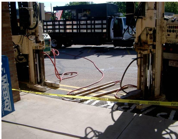
Figure 2. Direct injection outside of former dry cleaner.
