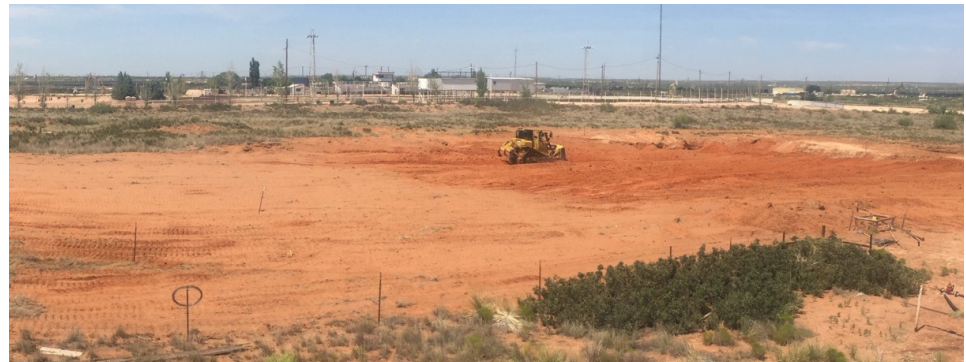
Figure 5. Panoramic View showing near Final Backfill of both Pit and Vent Excavations
