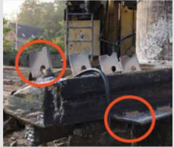
Figure 4. Discharge capability along the auger flights to convey grout to mixing zone
