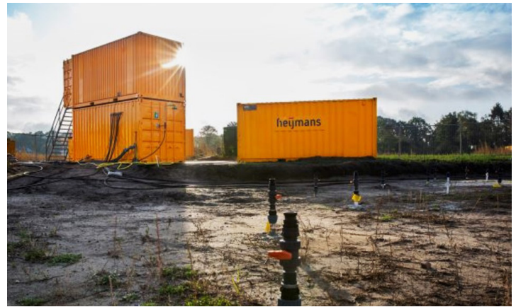
Figure 2. Injection Well Manifold
