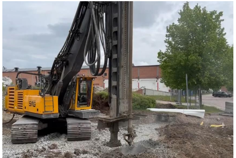
▲ SMG applying a blend of Klozur® SP and Portland Cement to the impacted area using large diameter augers.
