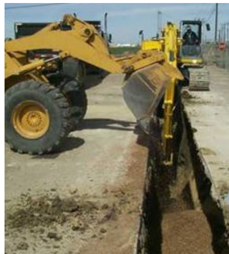
Figure 2. Placement of a mixture of EHC and sand into a trench excavation to form a PRB for plume control
