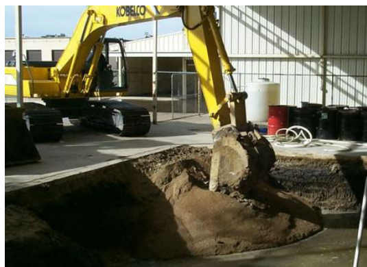
Figure 1. Backfill with 5% EHC by weight at an open excavation following source area removal
